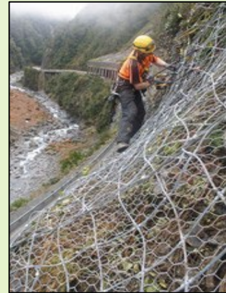
Loose rock confinement
