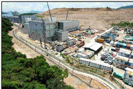
Desalination Plant at TKO 13/WSD/17, August 2023
