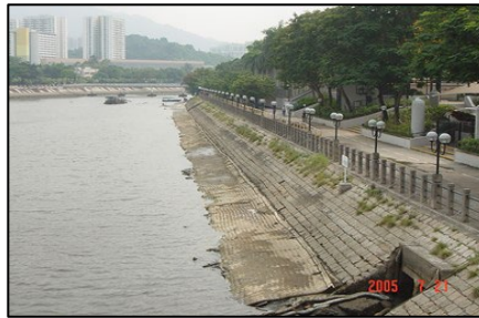
Shing Mun River scouring protection, July 2005
