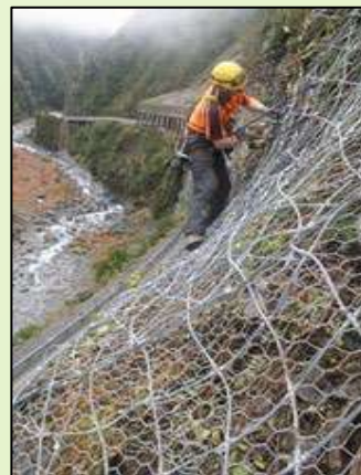
Loose rock confinement
