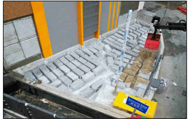
Water Retention Box PHD at Wang Chiu Road, January 2026 (HKHA20210526)
