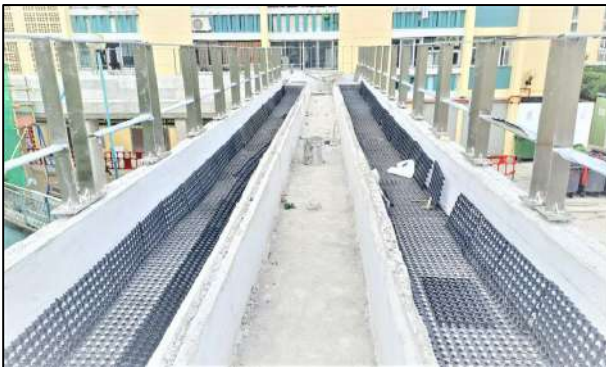
Planter drainage at Ching Hong Road August 2023 (HKHA20190687)
