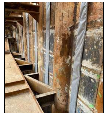
Basement Drainage Network Kwun Tong, March 2021
