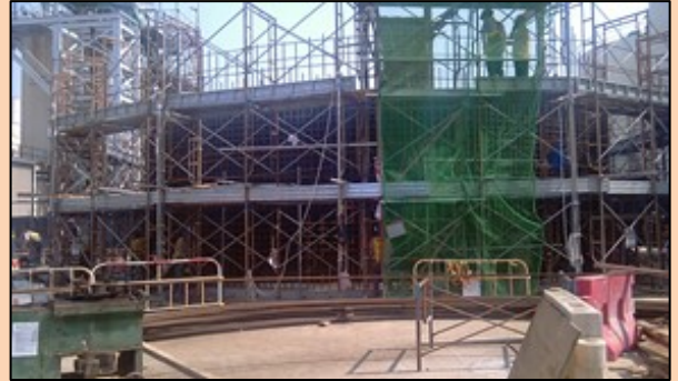
HAT Scheme Stage 2A, Upgrading Works at Stonecutters Island Sewage Treatment Facilities, DC/2009/17, October 2011
