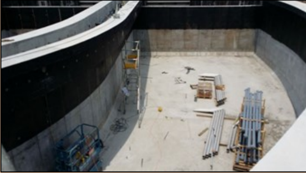
HATS Stage 2A, Upgrading Works at Stonecutter Island Sewage Treatment Works, DC/2009/10, May 2015
