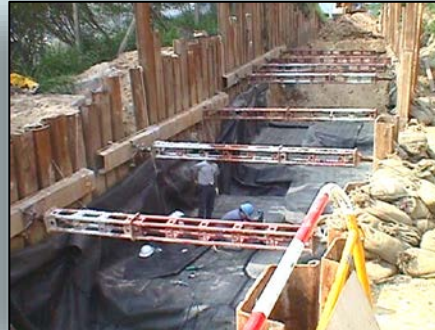
Leakage collection at Yuen Long, May 1999
