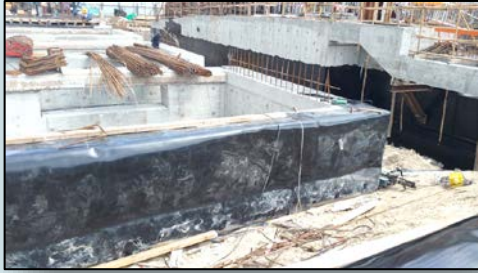
Tseung Kwan O Data Center, September 2015
