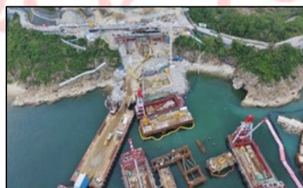
Hybrid system attached to work platform (NE/2015/01 & NE/2017/01)
