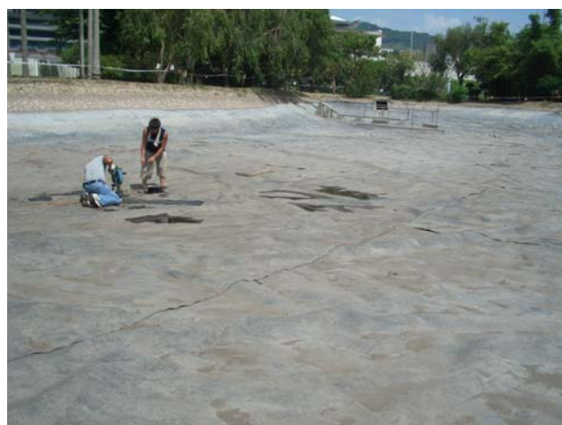
Repairing the Membrane, Sep 2005. Minor Repair Works were Necessary After Bobcat Operation.
