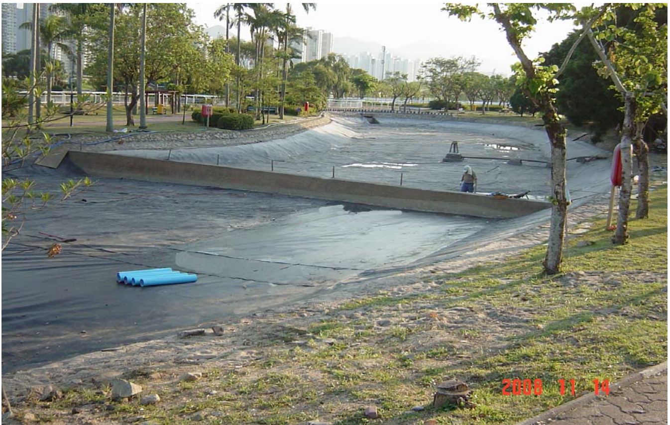
Addition of Sediment Separation Bund Repair Work After Construction Work in Existing HDPE Membrane.
