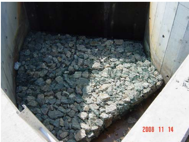
Filling Gabion with Rocks Along the Turn and Completion of First Layer
