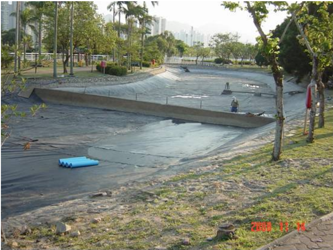
Addition of Sediment Separation Bund Repair Work After Construction Work on Existing HDPE Membrane
