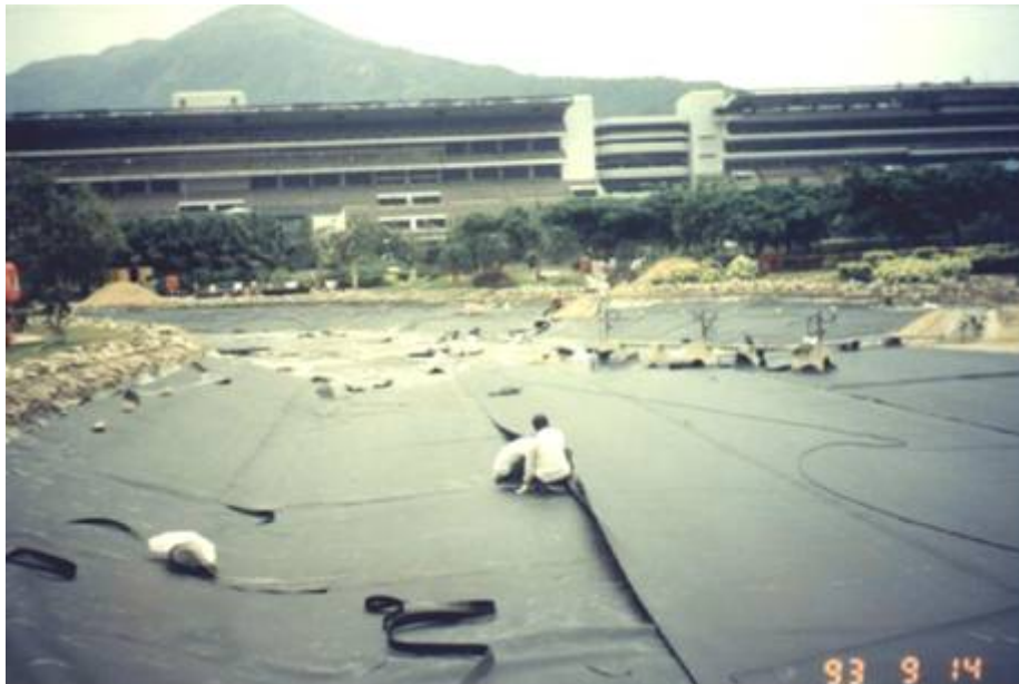
Laying Down of HDPE Membrane Waterproofing System at the bottom of pond, Sep 1993
